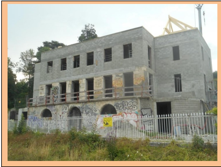
5 th stage: Assembly of the framework by journeymen. Fabrication of the roofs of the 2 towers on the ground
